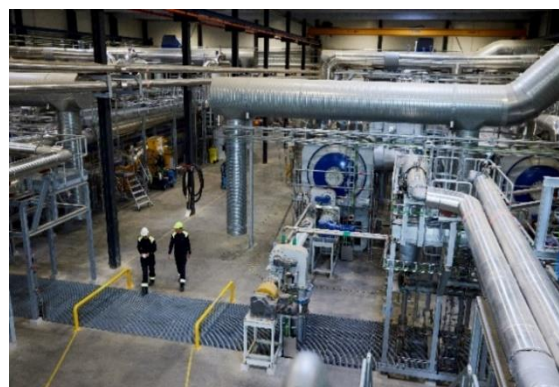
A reactor train in Skive
